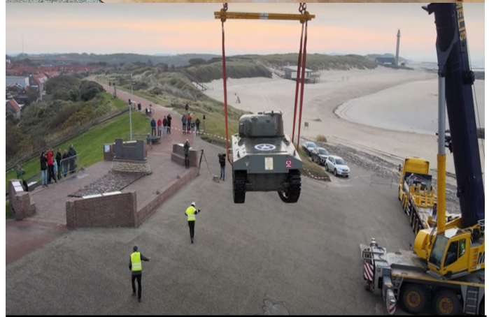
Westkapelle, Walcheren 18 October 2021: After a considerable restoration project, the Sherman tank was placed back on the stand overlooking the gap in the dike wall through which it had arrived as part of the assault force on 1 November 1944.
